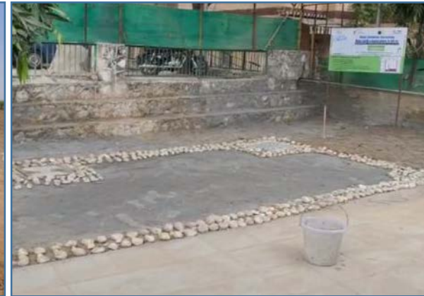
As part of PFS CSR initiatives, it has funded 25 sustainable Rain Water Harvesting structures in public/RWA parks and 25 Rain Gardens in Delhi NCR.
